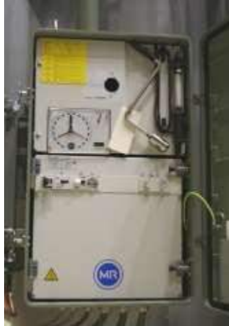
Modern tap changer of a transformer.
